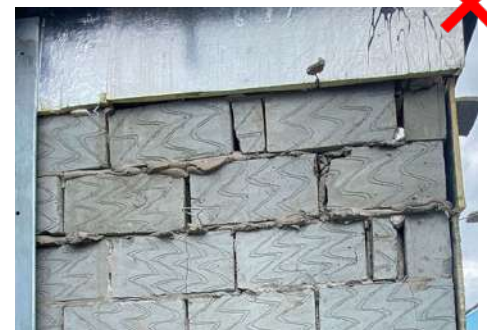
Unstable blockwork showing signs of movement/ cracking, requiring investigation
