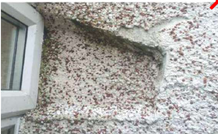
Badly cut out system to allow window to open
