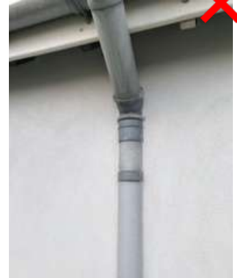
Pipe buried in render
