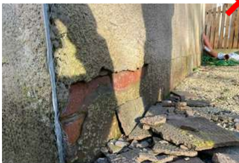
Substrate requiring investigation/ remedials prior to EWI installation
