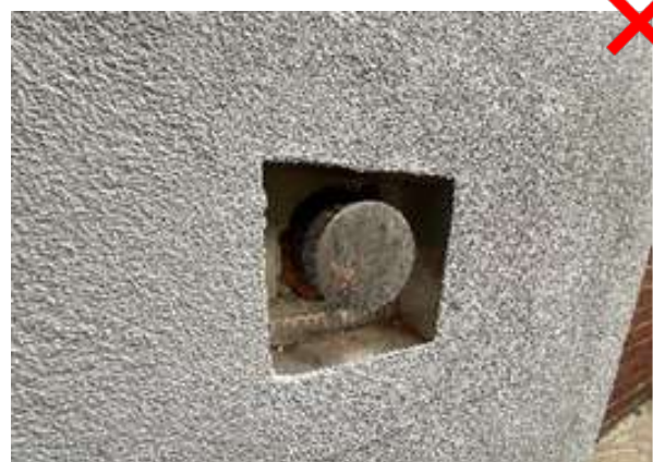
Non-extended flue with inadequate air flow
