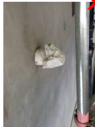
Flues should never be blocked
