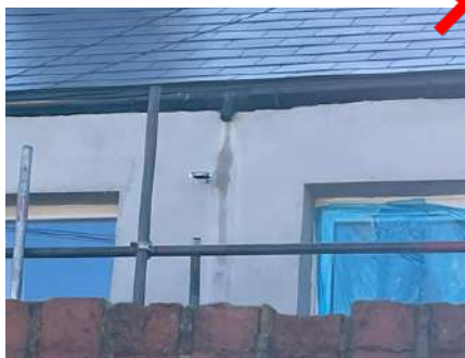
Inadequate protection allowing water to streak down and damage newly installed system
