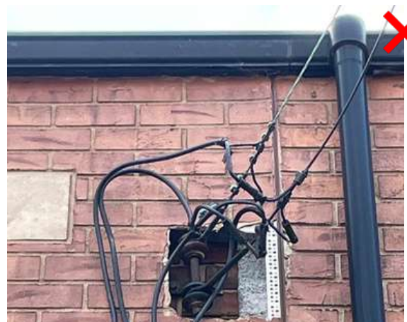
System left open around cables
