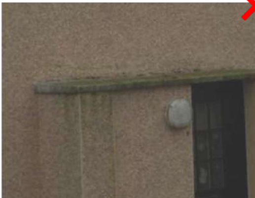
System finished on top of flat canopy with no protection to areas below
