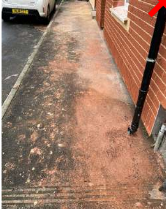
Inadequate protection of surrounding surfaces
