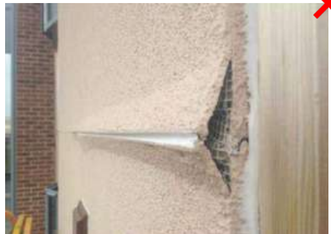
Excessive substrate movement
