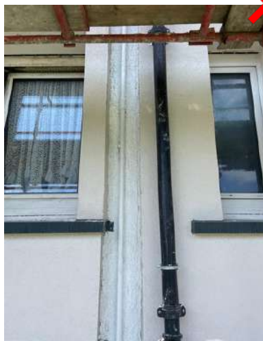
Uninsulated area around pipe causing cold bridge
