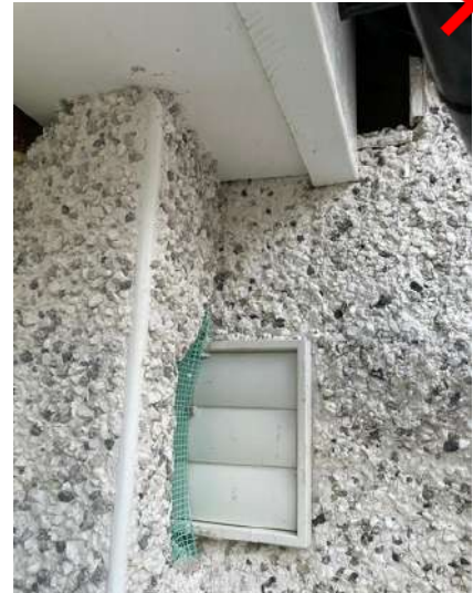
Vent buried in system
