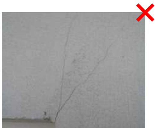
Cracks caused by no scrim patches installed
