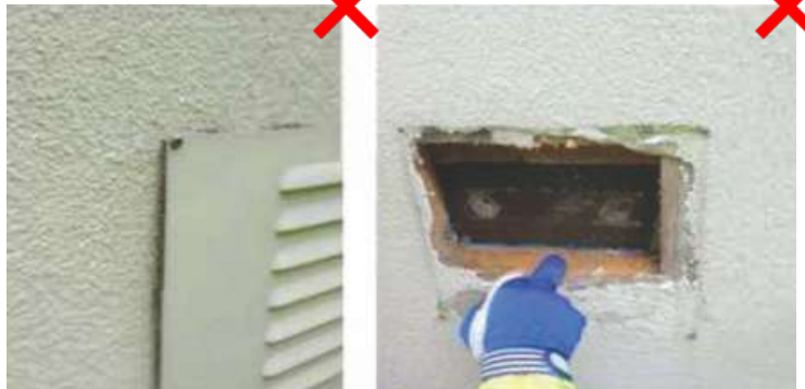
Vents not sealed, resulting in water ingress
