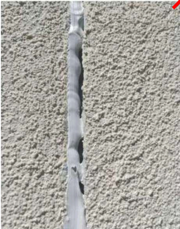
Movement Joint created with no beads and incomplete mastic, allowing water ingress
