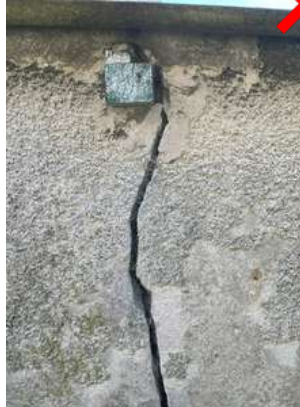
Structural movement requires investigation and should not simply be insulated over
