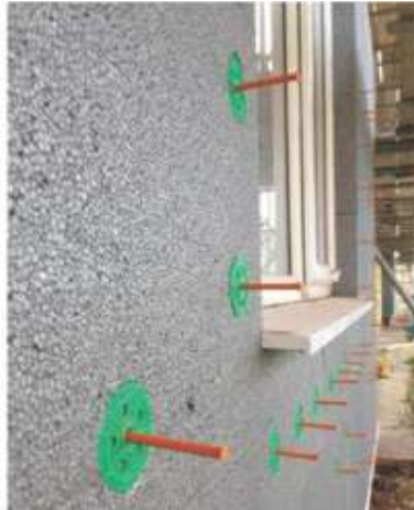
New Cill with Correct Overhang
