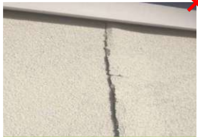
Movement causing cracking where no movement joint is installed
