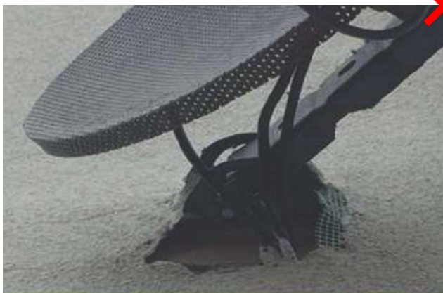
Satellite dish install completely incorrect
