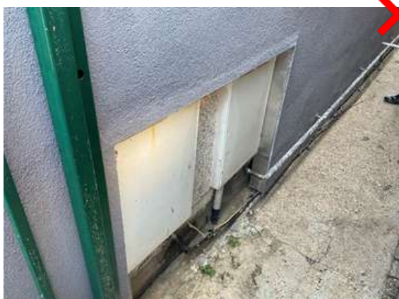
Large cold bridge around gas boxes
